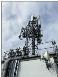
TELECOMS ARE ROOF MOUNTED ON PLANT ROOM.
