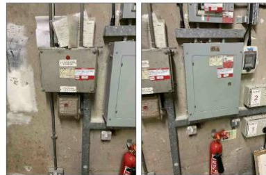
MAINS & LIFT ISOLATORS WITHIN ROOM MOUNTED PLANT ROOM.
