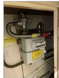
GAS METERS & ISOLATION POINT.
