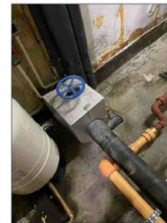
MAINS COLD WATER ISOLATION POINT.
